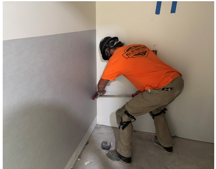
Bouten Construction installing wall protection in Area C within the Wellness Room.
