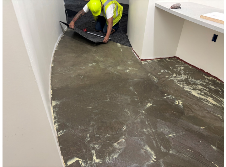
Standard Paint & Floor installing carpet tile within the Control room of Area A.
